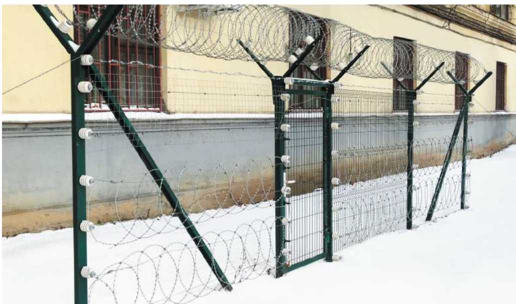
Model of the system "KRAPIVA" installed in the testing ground
